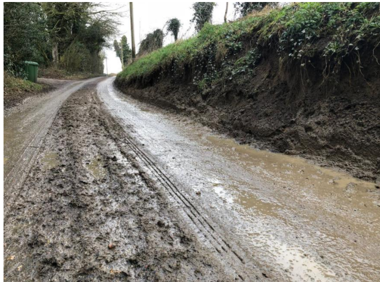
Photograph: Collapsed bank along Mergate Lane - metres away from Barracks Meadow.
