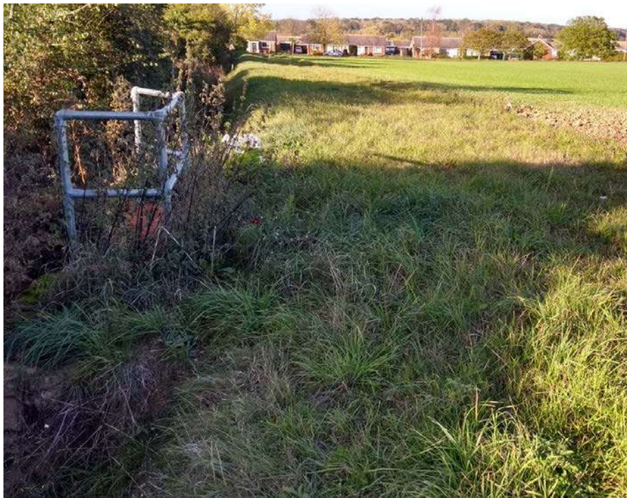
Image showing the Harvest way development outfall to the western boundary ditch, looking north towards Green Lane
