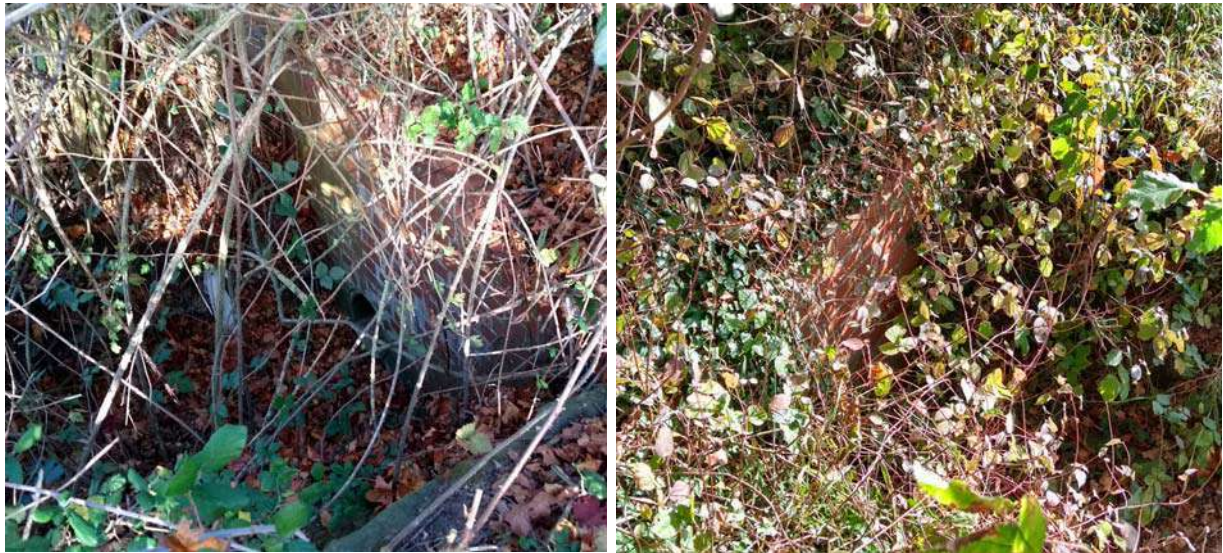
Headwalls at the heads of the two Green Lane watercourses/drainage ditches to the west of the A 143 (north of Green Lane on the left, south of Green Lane on the east)
